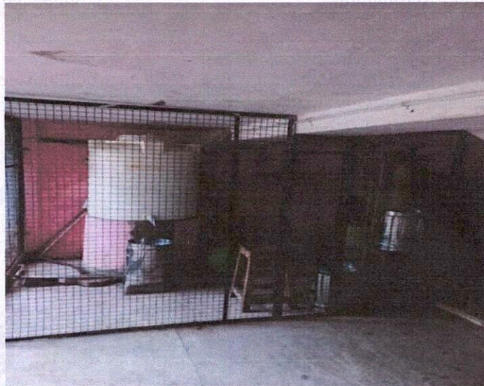
R.O. Water Plant installed in our college campus.
